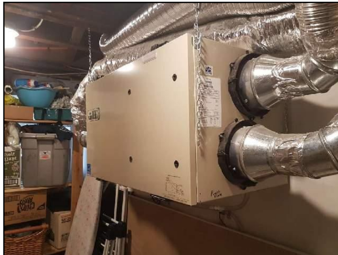
8. Heat recovery ventilator (HRV)
