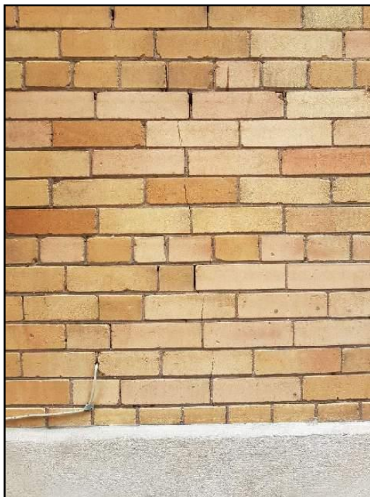
3. Typical minor cracks, not structurally...
