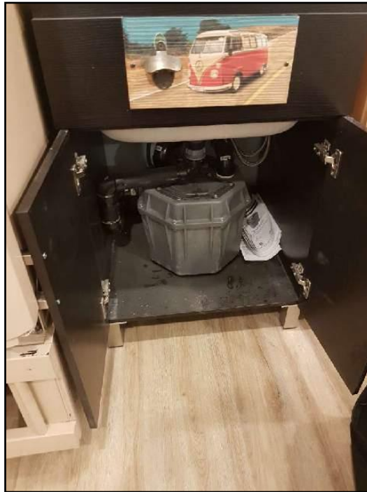
10. Laundry tub pump
